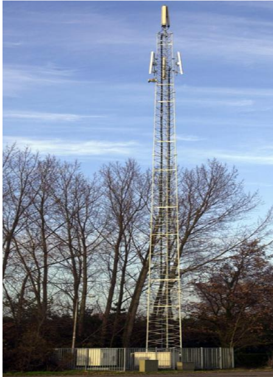
cellular base station
